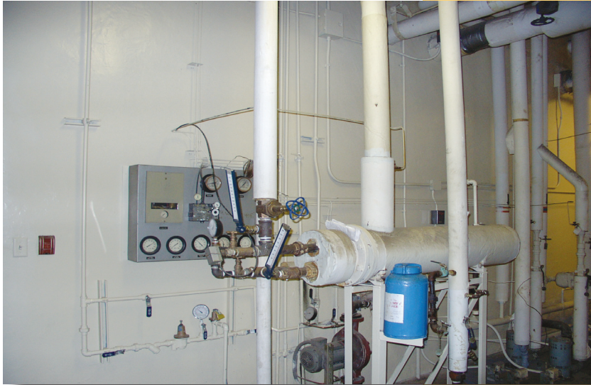
Heat Exchanger in use
